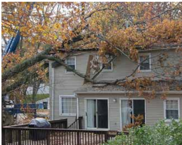
Photo 1—The high winds of a storm like Sandy can push over trees into homes, cars, and utility poles. Even in areas with underground utilities, above ground power lines can still be broken, causing local electrical blackouts.
