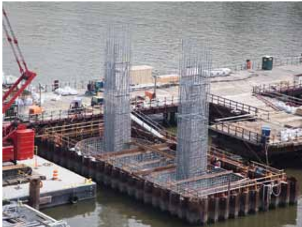
Photo 5 (below)— The first pier columns are being erected on top of one of the completed piers.
