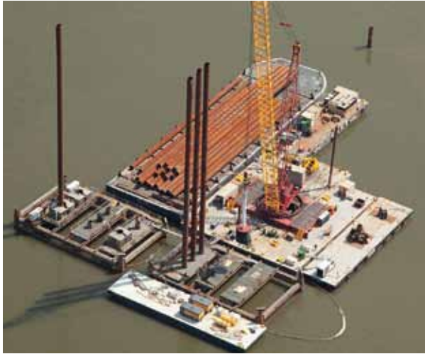
Photo 4 (left)— These giant, hollow steel tubes were pile driven down through the silt to the bedrock.
